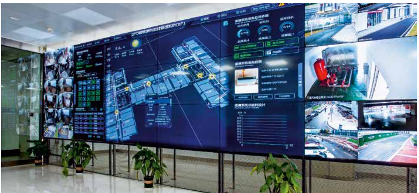
The building management system incorporates all relevant sub-systems. © Dongfeng Design Institute
