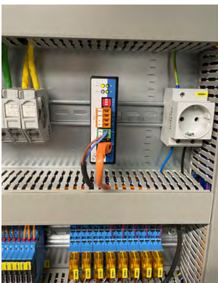
A UBR-01 is used at every KMG Kliniken site. Integration took place in the existing system – during ongoing operations.
