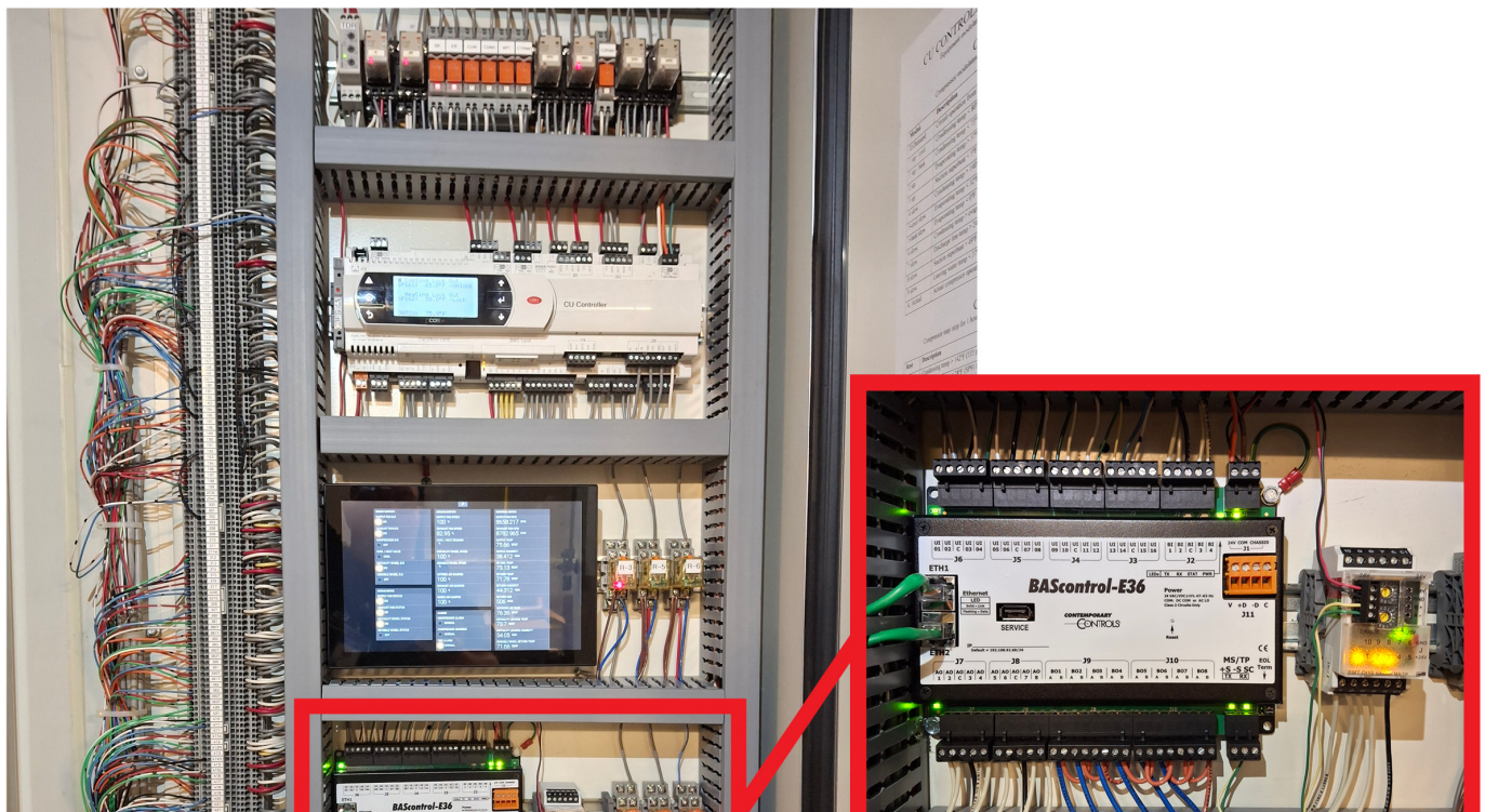
Control panel showing the final system architecture, featuring a BAScontrol-E36 primary controller, MS/TP-connected I/O expansion module, and touchscreen interface to monitor and regulate compressor modulation for the outdoor air units.
